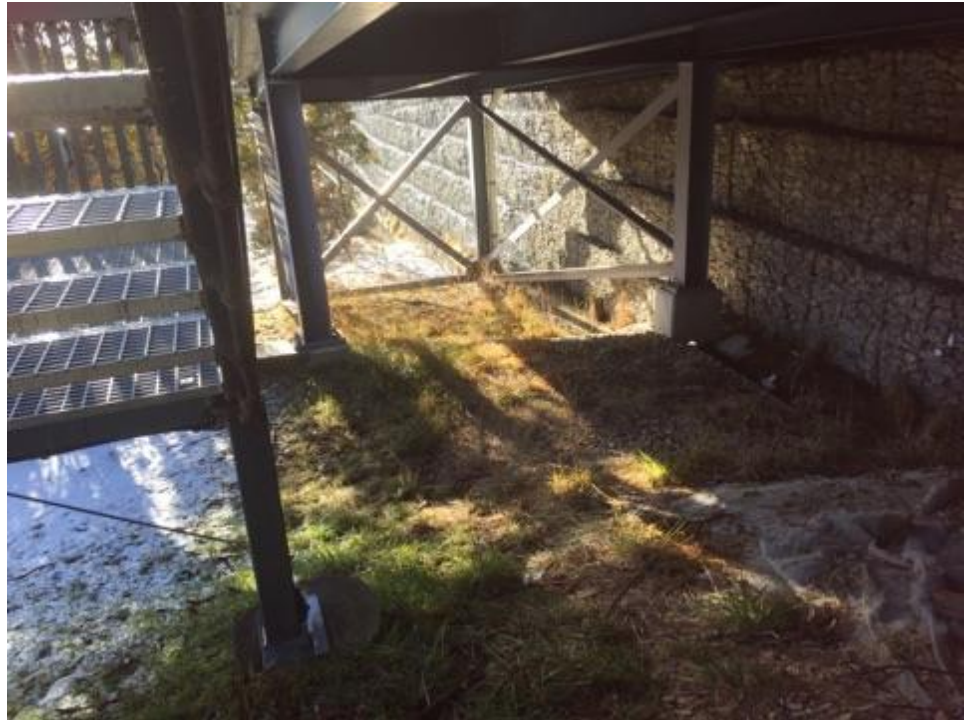
Figure 7: Photo of the are to be enclosed as a bike storage area
