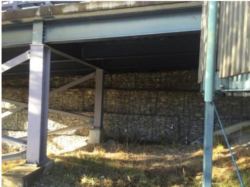
Figure 9: Photo of the are to be enclosed as a bike storage area showing area to be paved
