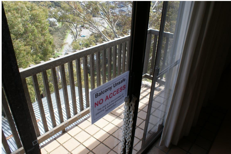
Figure 5: Photo of the existing balcony to be demolished and Aneeki's roof below
